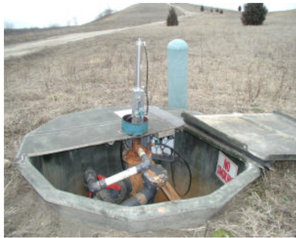
The Anchor Pump 102A in the vault with the dome.
