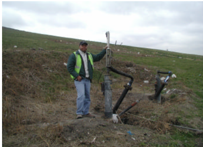
Tony Brooks, Leachate Technical Supervisor, shown here with one of the 31 Blackhawk Pneumatic Anchor Pumps.
