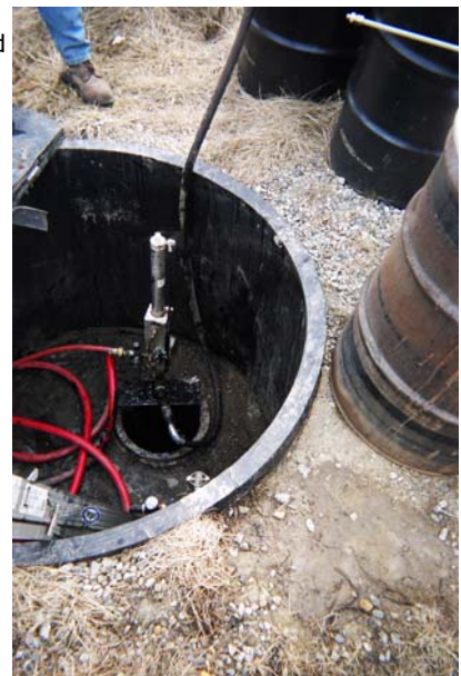
Blackhawk Pneumatic Pump is relatively maintenance-free even after pumping tar pitch at oil refinery site.
