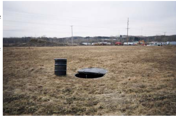
Tar refinery site in Ohio where Blackhawk Pneumatic Pumps are pumping tar pitch.
