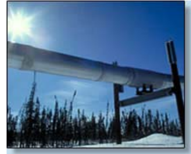
The pipeline shown here is typical of those being used by this US Fortune 500 gas and power marketer.
