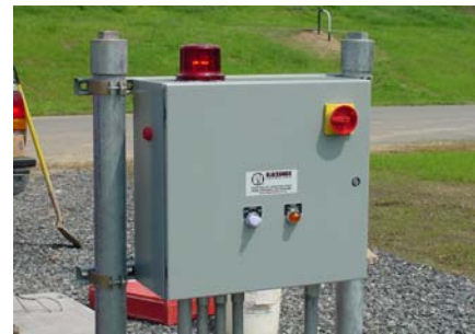
Electric Control Panel for Blackhawk Pump at Salem County Utilities Authority Landfill.
