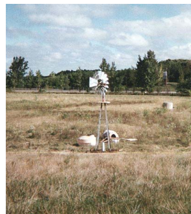
Blackhawk Windmill Pumps operate successfully in many landfills pumping from 500—1500 gpd.
