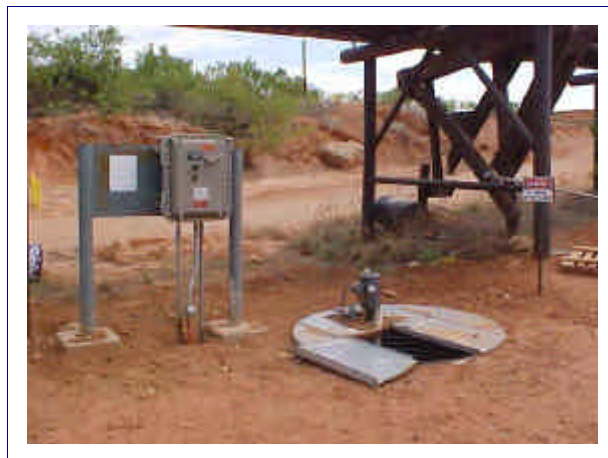
Blackhawk Explosion-Proof Electric Anchor Pump pumps old extremely flammable viscous petroleum byproduct 24 hours/day.
