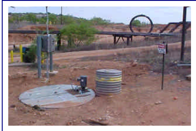
Blackhawk Explosion-Proof Electric Pump and controls installed at the petroleum refinery.
