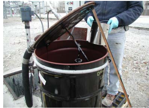
Gordon O'Toole, MTR Consultants (Management & Technical Resources, Inc.) opening one of the 55 gallon drums of thick, viscous, oily and sticky coal tar that was pumped from 32 feet underground using Blackhawk's electric Anchor 101 pump.
