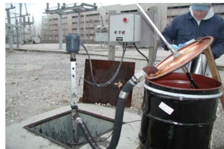
An average of three 55 gallon drums of coal tar are pumped each month from these two wells using Blackhawk electric Anchor 101 pumps at the South Carolina Electric & Gas Superfund site in Charleston, SC.
