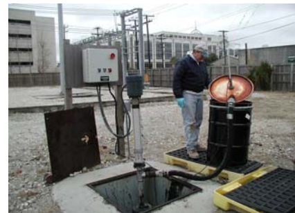
This Blackhawk electric Anchor 101 pumps extremely thick and heavy coal tar from 3 feet underground at a controlled rate of one minute every hour around the clock.
