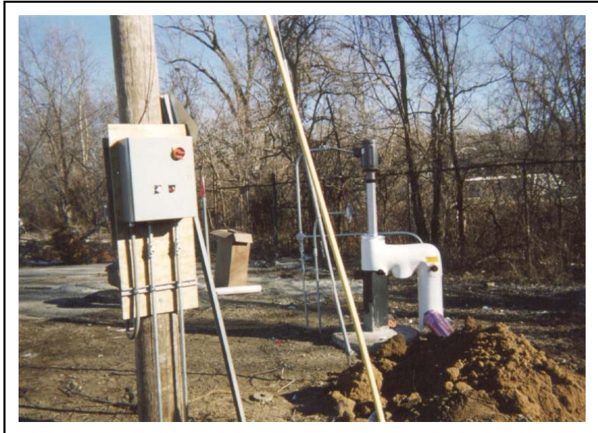
Control box for one of the four Blackhawk Electric 102 Anchor Piston Pumps working 24/7 at BP Sugar Creek site.
