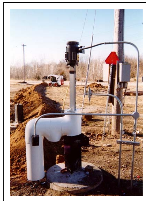
One of Blackhawk's 102 Electric Anchor Piston Pumps controlling and containing groundwater from migrating into Sugar Creek.
