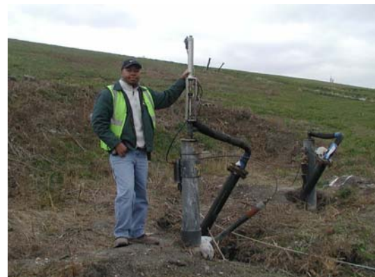
Tony Brooks, Leachate Technical Supervisor, shown here with one of the 31 Blackhawk Pneumatic Anchor Pumps.
