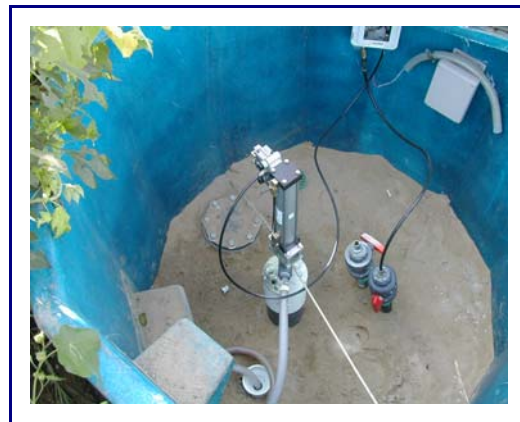
Blackhawk's Pneumatic Trident Pump, housed in a 4-foot vault to conceal it from view, continually pumps the accumulated stormwater runoff into a 10,000-gallon collection tank.
